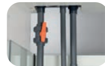
Pipework pre-assembled: Fixed pipework made of PVC-U; silicone hose as coupling piece to the feed pump (plug & play system)
